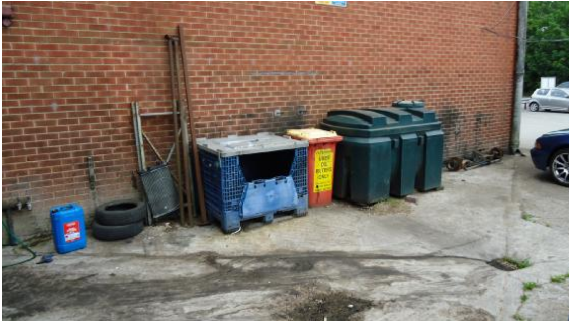
AST, old oil filter bin and other items including evidence of potential contamination migrating into the drainage system.
